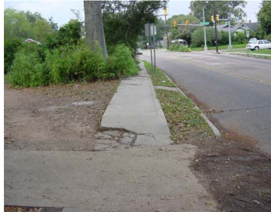
A sidewalk on Voorhies St. that is in need of maintenance.
